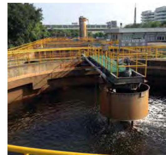
Effluent Treatment Plant at LWG-Gold-certified PUMA Leather Supplier Prime Asia
