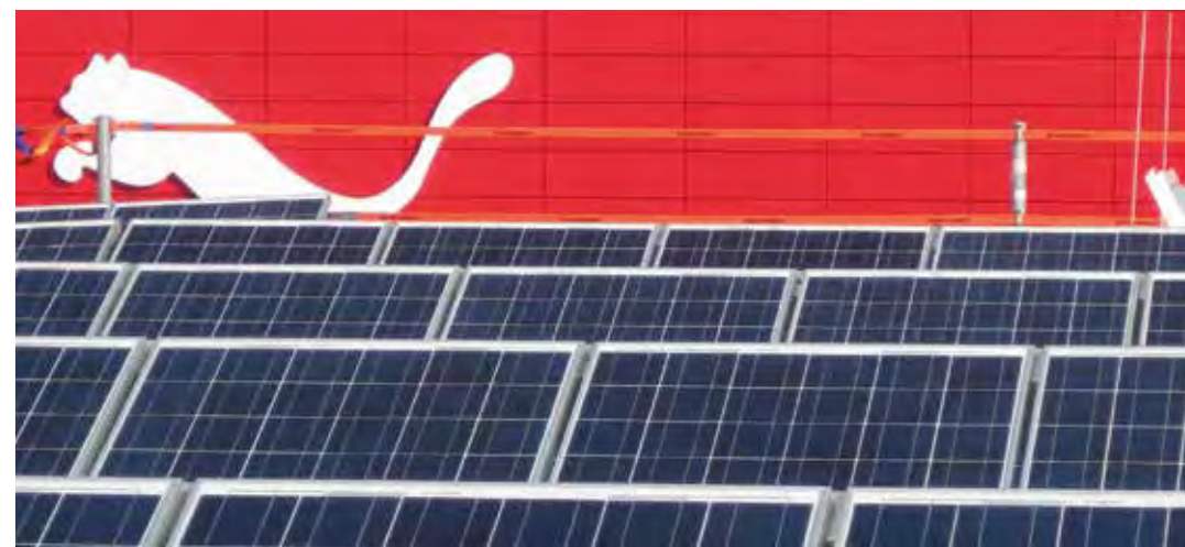
Solar panels on the roof top of PUMAVision Headquarters in Herzogenaurach, Germany
