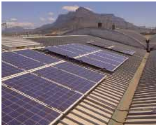
SOLAR POWER STATION for generating electricity on the roof of PUMA supplier factory Impahla Clothing, Cape Town South Africa
